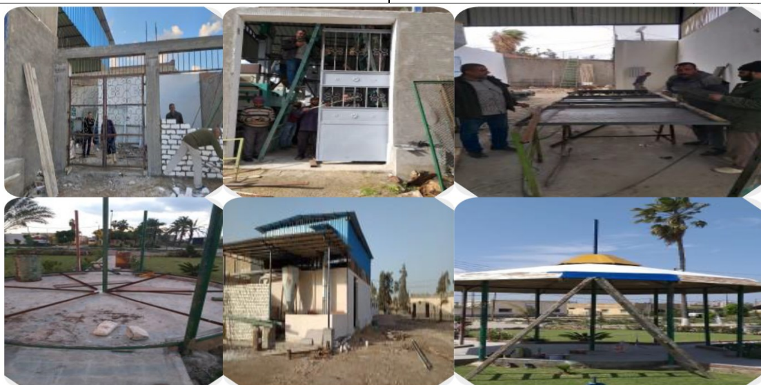
Recycling Program for both materials and equipment with metals and derivatives (Alexandria University, Egypt)
