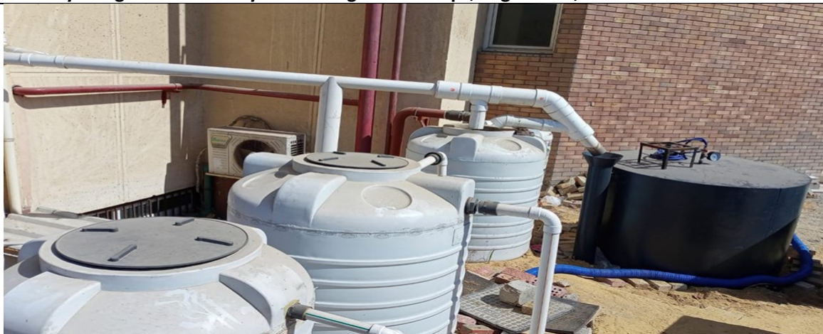
Wastewater treatment unit at Faculty of Engineering
